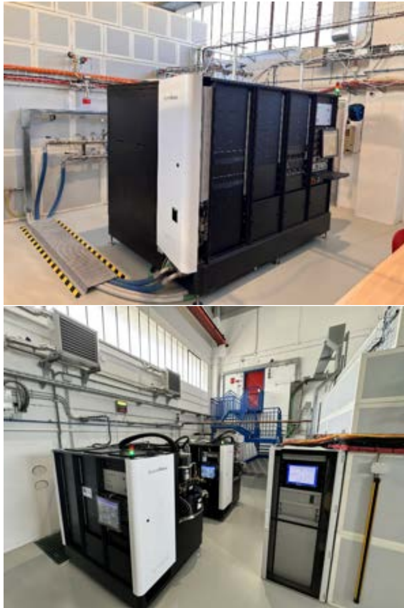
Figure 13.8: Picture of the solid-state RF sources at the TEX facility. In order X-band 50 MW, 50 Hz source, X-band 25 MW, 400 Hz source and C-band 20 MW, 400 Hz source.
